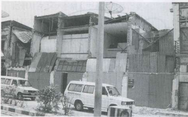
Damage by Earthquake at Pare-Pare
